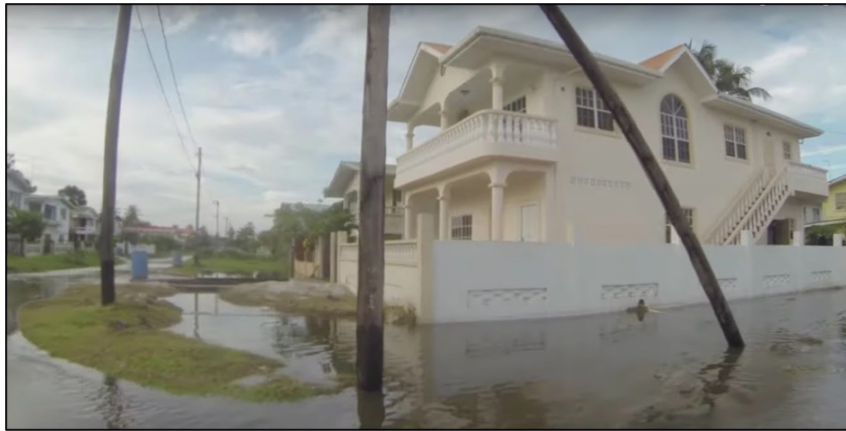
Figure 5 Screenshot of electrical poles in Georgetown becoming rotted by floodwater. From The Real Atlantis – Is Georgetown, Guyana a Sinking City? (7:18), by Real Guyana, 2013.
